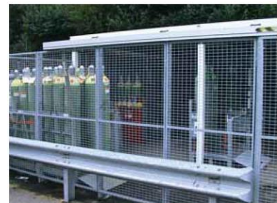
Figure 7: Fence protecting gas bottles Source: Suva
