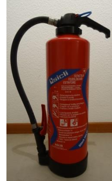
Figure 4: Fire extinguisher Source: CSD
