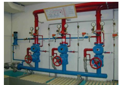
Figure 6: Sprinkler station Source: CSD
