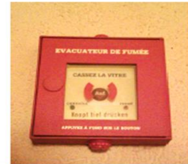
Smoke alarm (connection to fire brigade)
