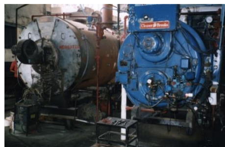
Figure 3-24: Fuel oil operated boilers [72]
