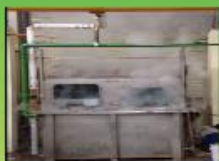
Obsolete dyeing equipment
