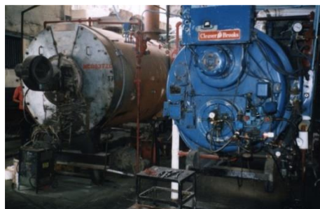
Figure 4-20: Fuel oil operated boilers [87]
