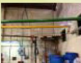
Steam system measures
