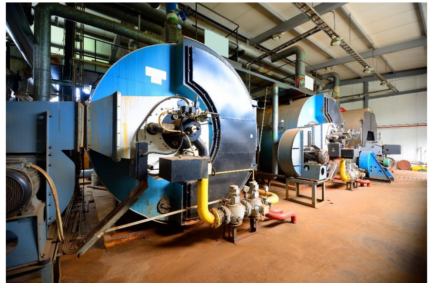
Industrial boiler room
