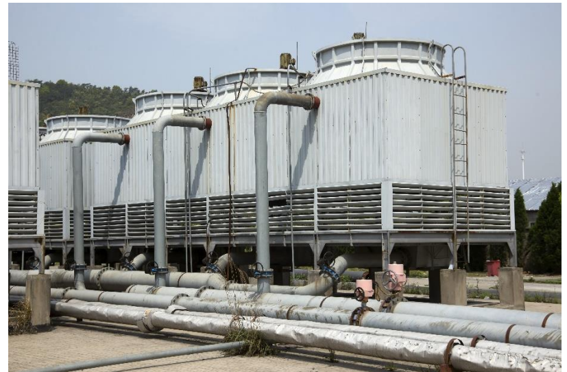
Cooling towers Source : Shutterstock
